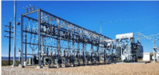
This part of the substation is where a huge transformer and wiring framework settled and needed underpinning.
