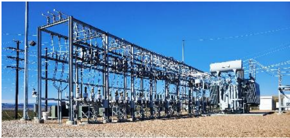
This part of the substation is where a huge transformer and wiring framework settled and needed underpinning.
