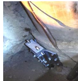
This is a view of a completed pier installation on a caisson.
