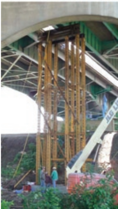
These photographs show the falsework in place under the bridge, the steel beams under the bridge girder and one of the concrete footings.
