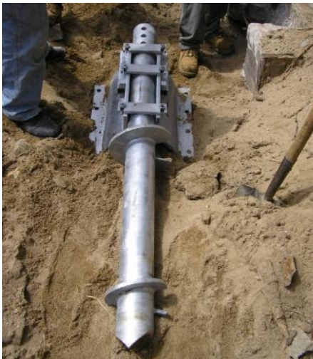
This photo shows the configuration of the helical pile and custom bracket designed by ECP.
