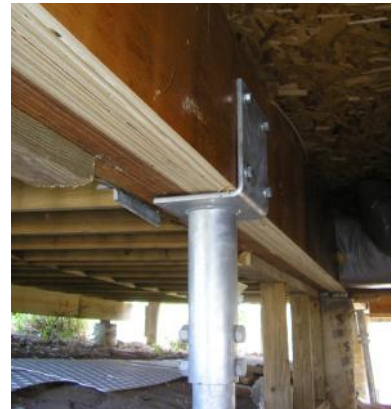
The photographs above show the pile installations being completed in the tight conditions under the structure.
